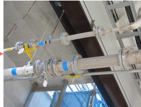
ヘリウム回収配管 Recovery Piping (Low-pressure than atmosphere)
